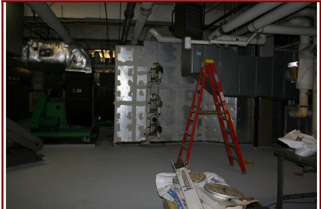
VIEW OF MECHANICAL AREAS
