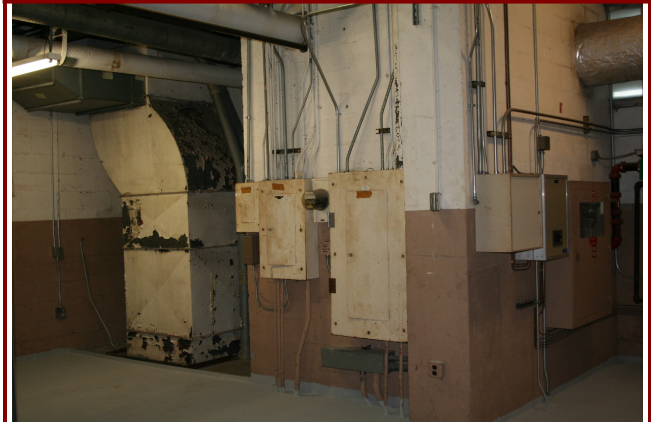
VIEW OF MECHANICAL AREAS
