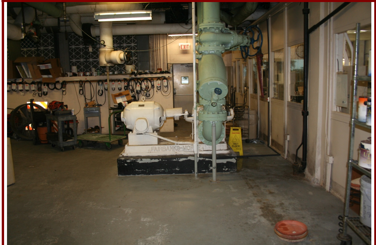
VIEW OF HVAC PLANT
