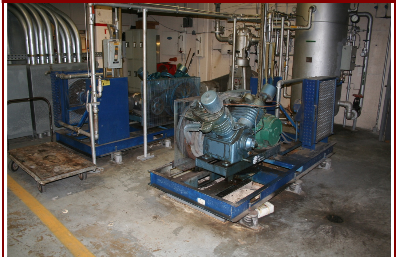
VIEW OF AIR COMPRESSORS
