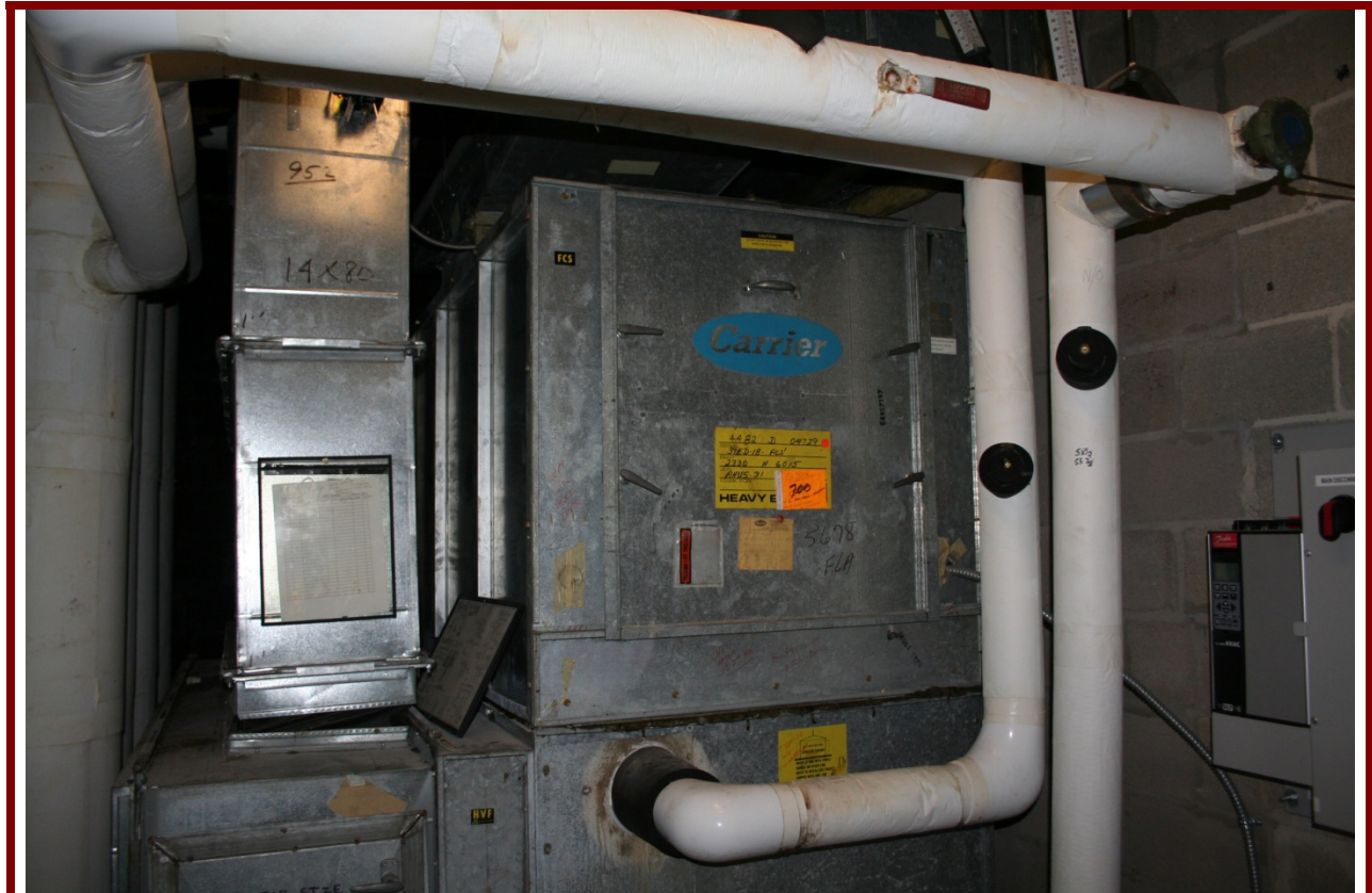
VIEW OF REPRESENTATIVE AIR HANDLER
