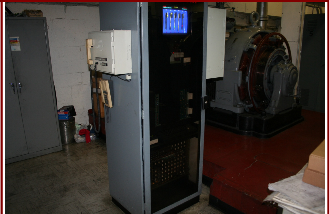
VIEW OF REPRESENTATIVE ELEVATOR CONTROLLER AND WINCH HOIST
