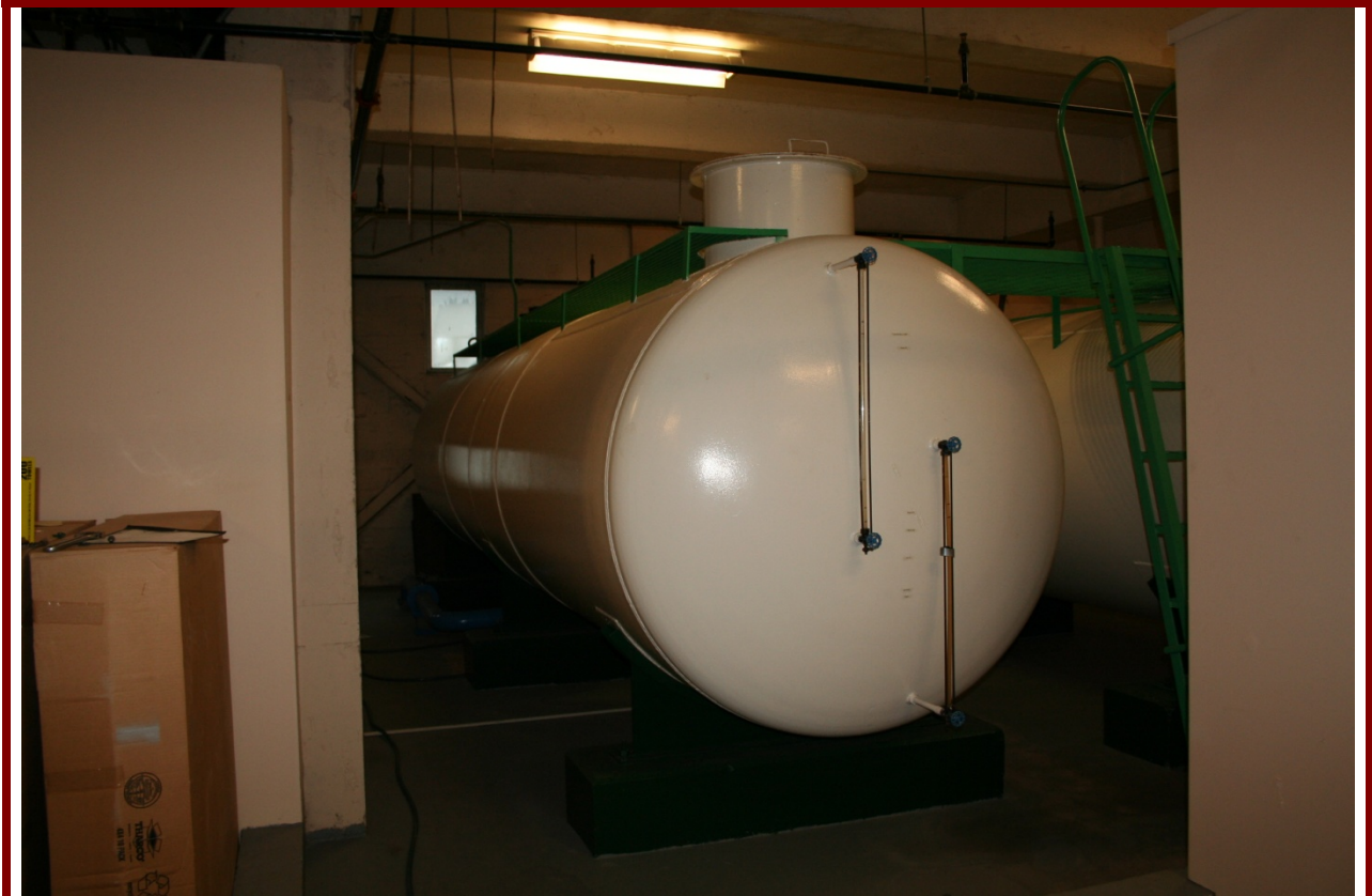
VIEW OF DOMESTIC WATER HOLDING TANK 6-23 FLOORS
