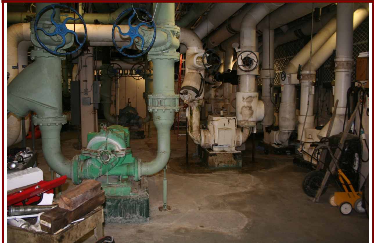
VIEW OF HVAC PLANT
