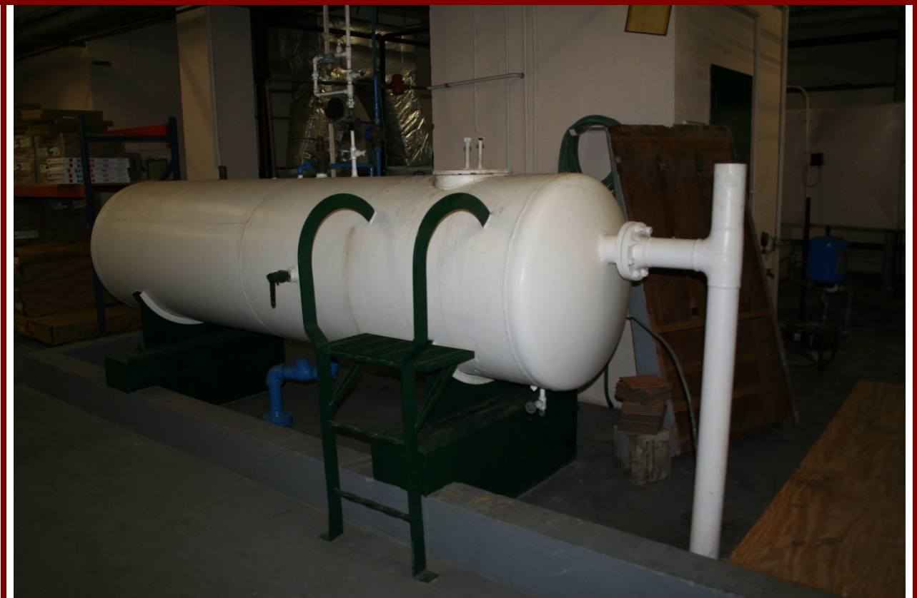
VIEW OF MECHANICAL AREAS
