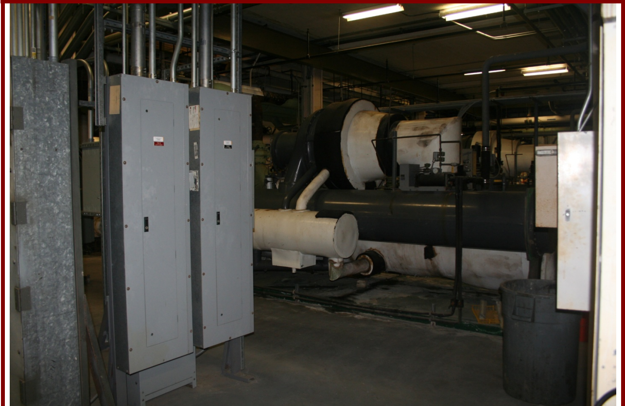
VIEW OF HVAC PLANT
