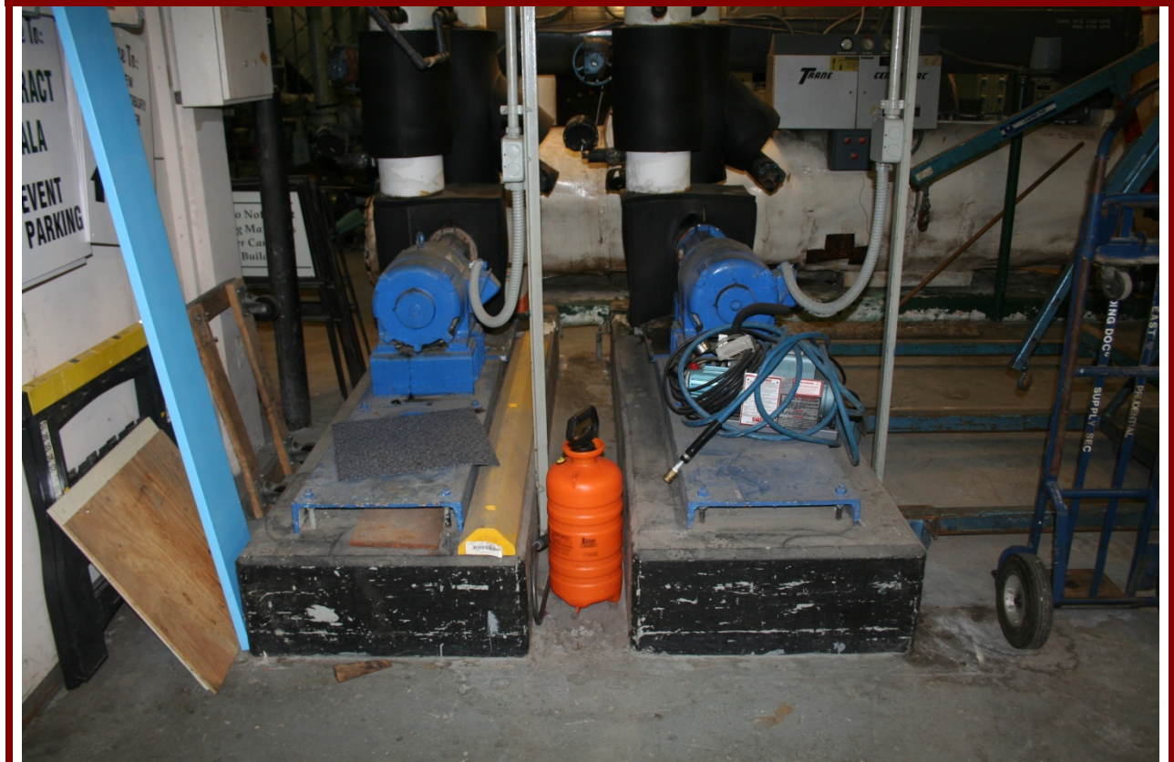
VIEW OF HVAC PLANT
