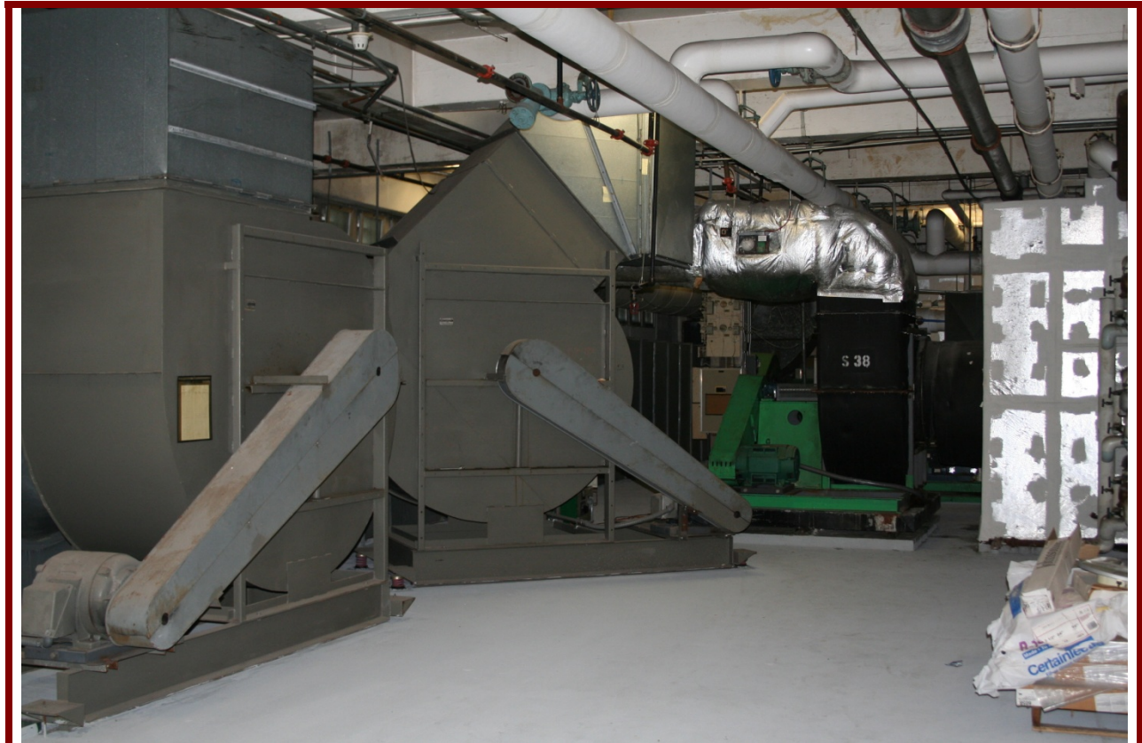
VIEW OF MECHANICAL AREAS
