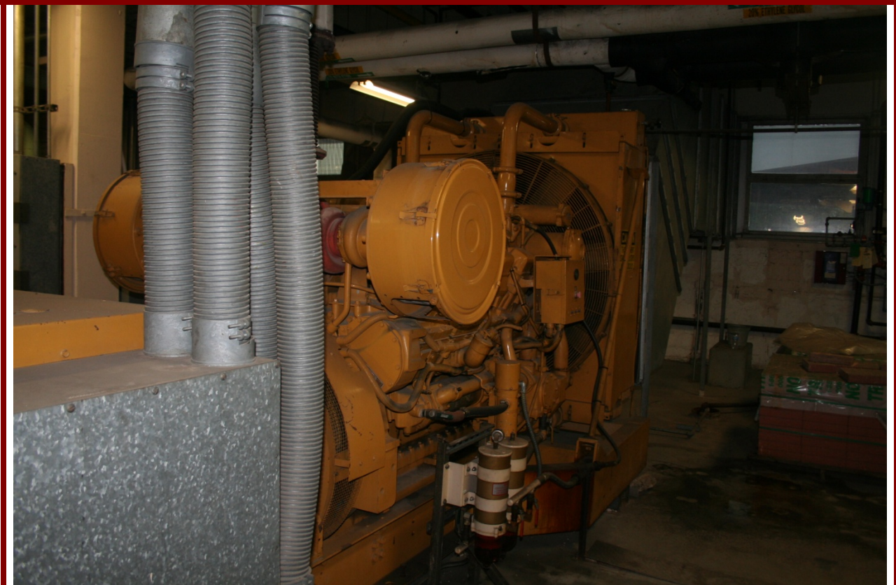
VIEW OF DIESEL ENGINE POWERED EMERGENCY ELECTRICAL GENERATOR
