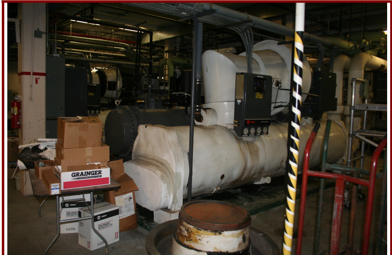
VIEW OF HVAC PLANT
