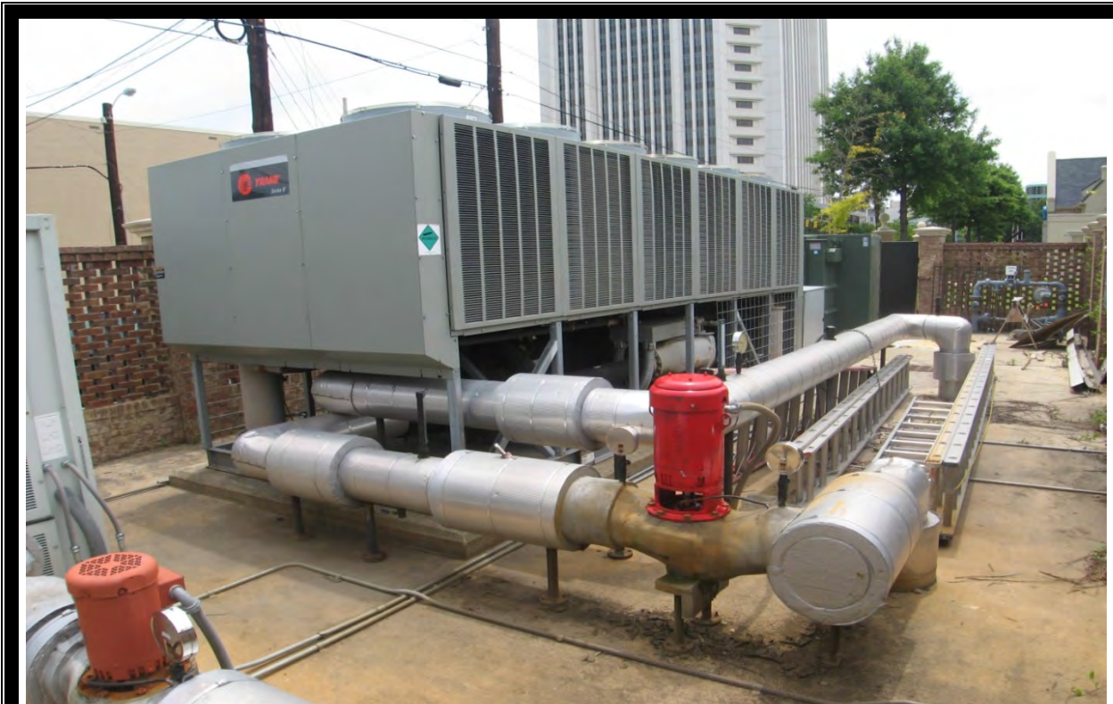
VIEW OF HVAC EQUIPMENT
