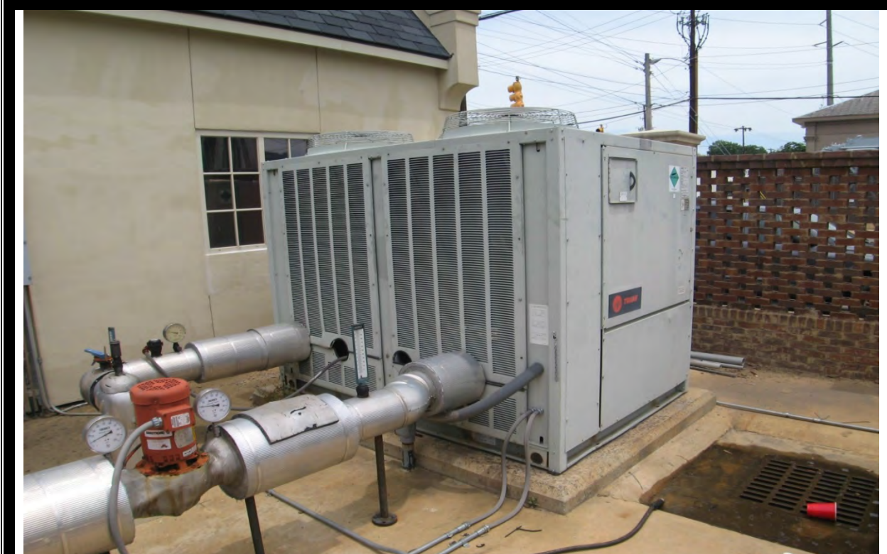
VIEW OF HVAC EQUIPMENT
