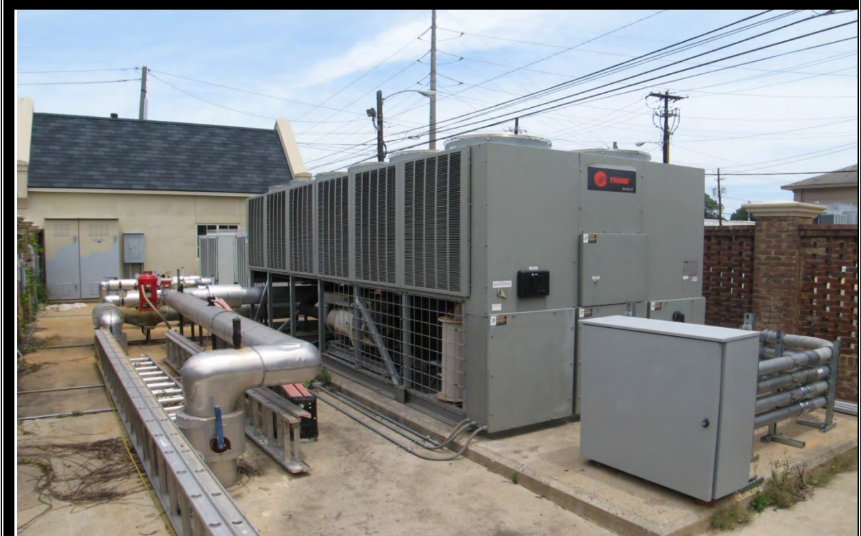
VIEW OF HVAC EQUIPMENT
