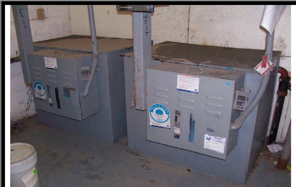
VIEW OF TYPICAL BUILDING MECHANICAL EQUIPMENT
