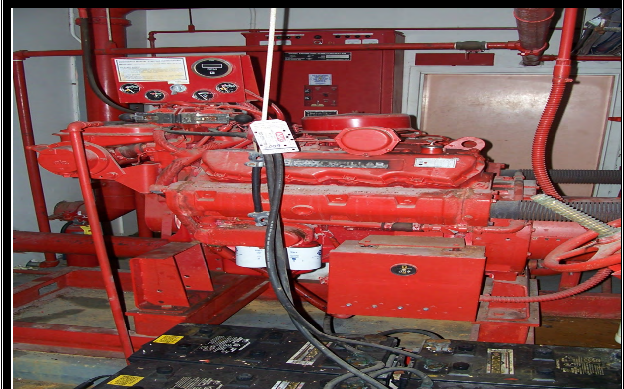
VIEW OF TYPICAL BUILDING MECHANICAL EQUIPMENT
