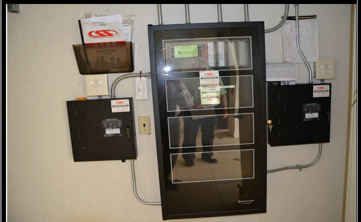
VIEW OF AUTOMATIC FIRE NOTIFICATION SYSTEM
