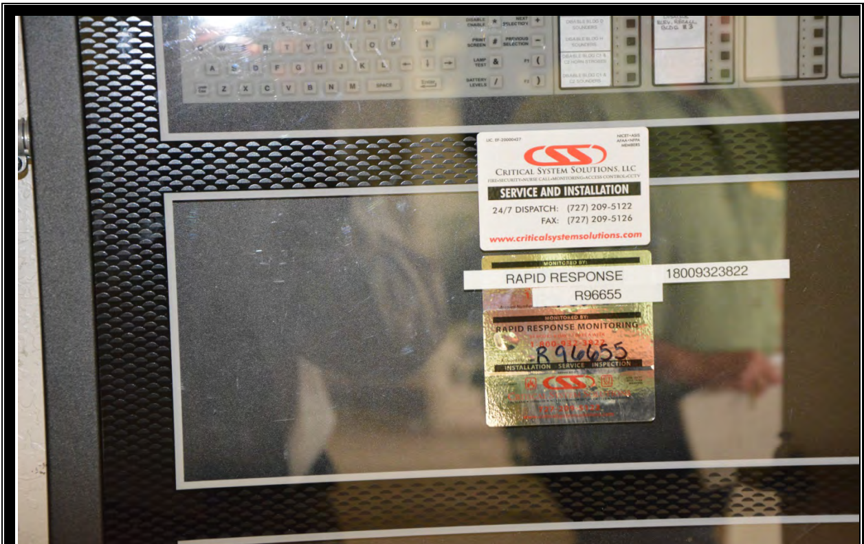
VIEW OF AUTOMATIC FIRE NOTIFICATION SYSTEM
