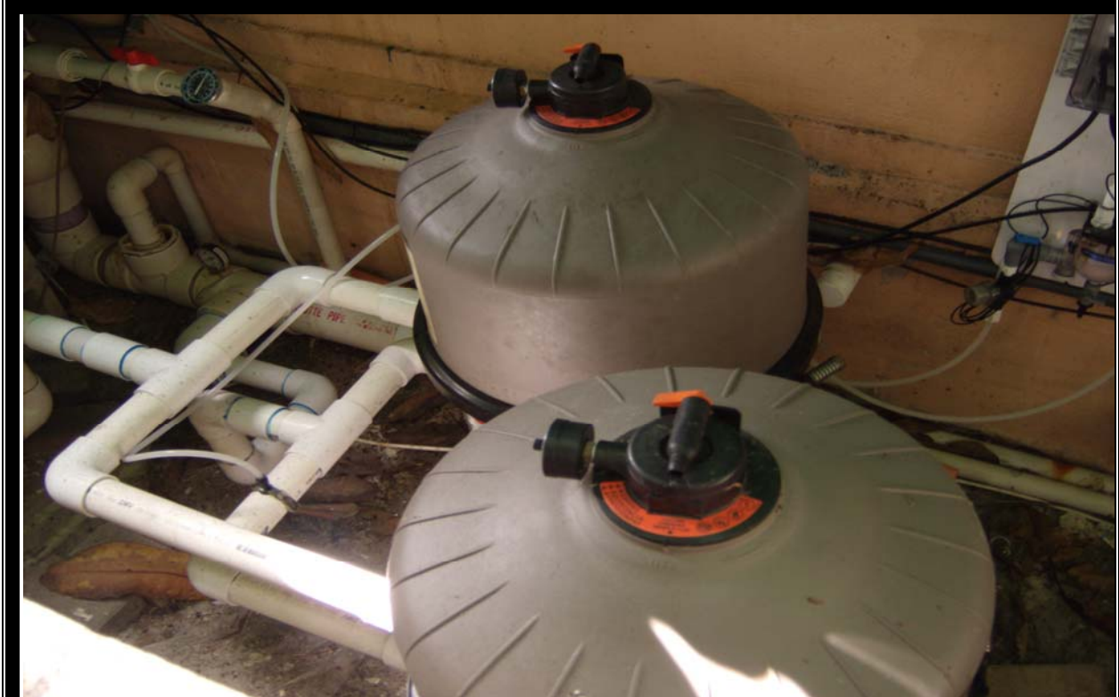
VIEW OF TYPICAL SWIMMING POOL EQUIPMENT
